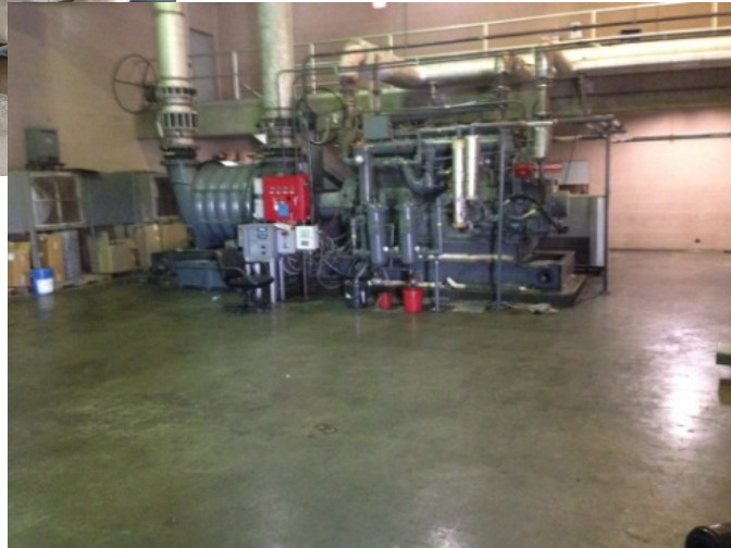
Engine and Blower with control panel
