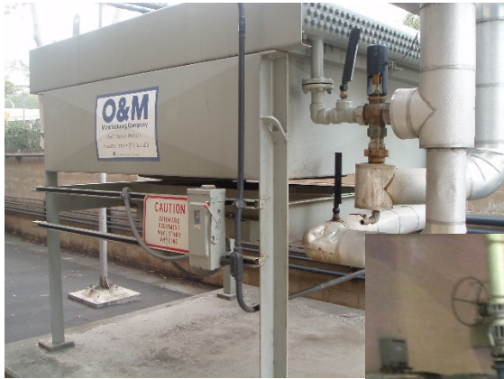
Once through waste cooling system
