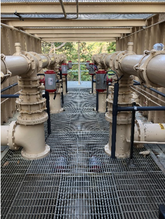
Figure 3 – New Air Tubing to Filter Valve Actuators
