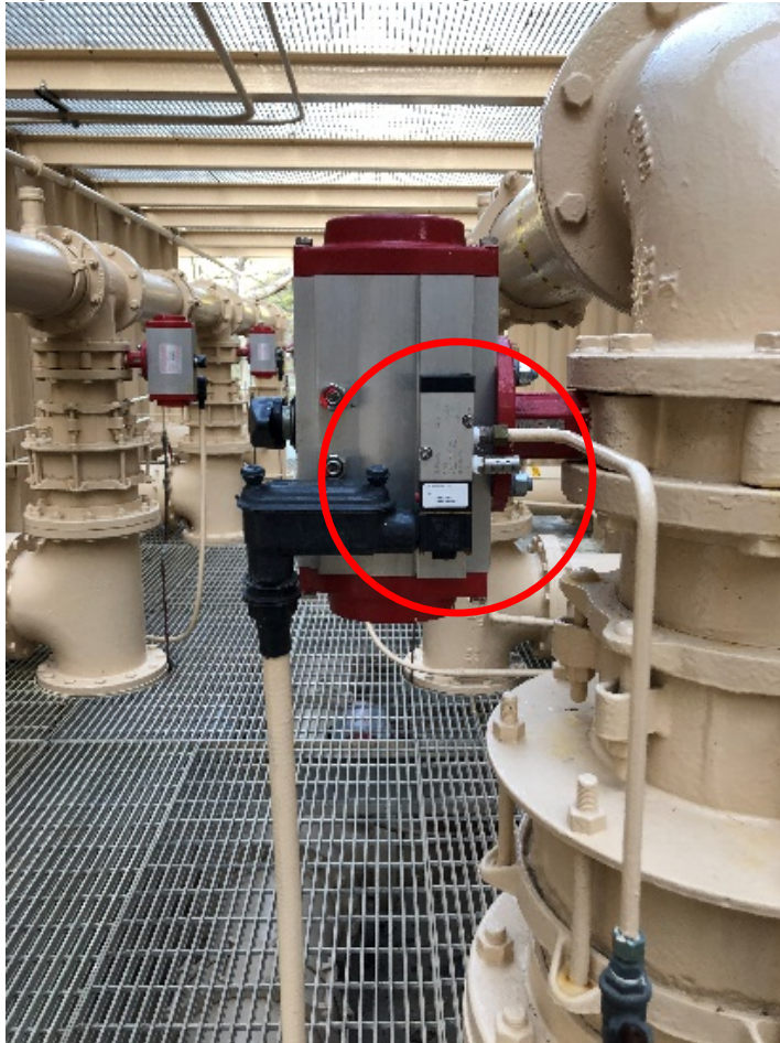
Figure 1 – Old Pilot Valve Configuration
