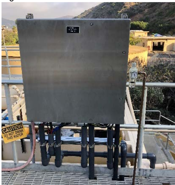
Figure 2 – New Valve Control Panel
