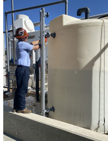
Bleach Tank sight-glass at RTP
