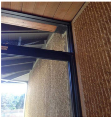
Photo 6: Glass Crack at Door 117
