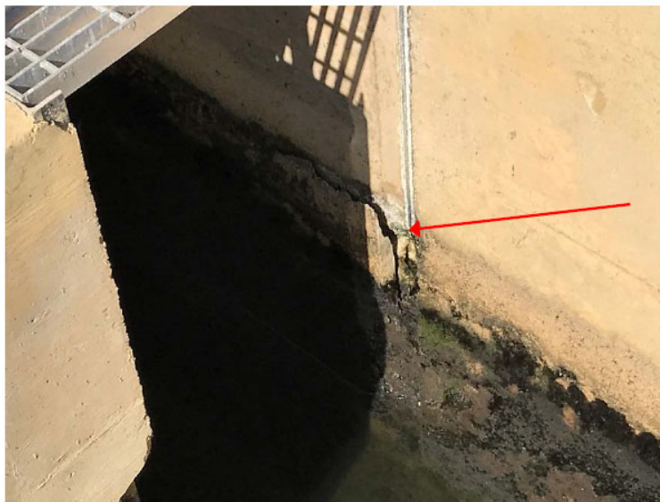
Figure 1.3 Concrete Spalling at Flocculation Basin Stop Plate Opening
