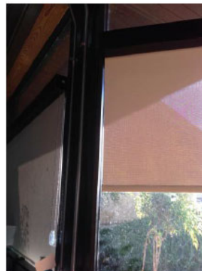
Photo 15: Bowed Mullion - Viewed from Interior
