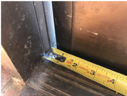
Photo 5: Gap Between the Window and Wall Frame at Door 117
