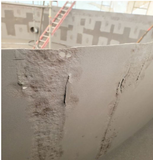
DAFT 2 Internal Corrosion
