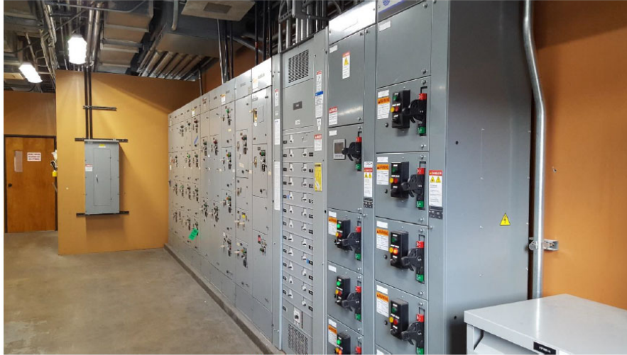
MCC-B AND MCC-H
