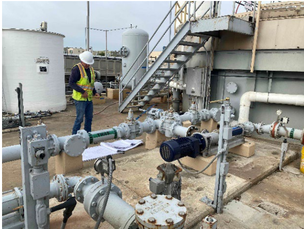
Existing TWAS Pump Station
