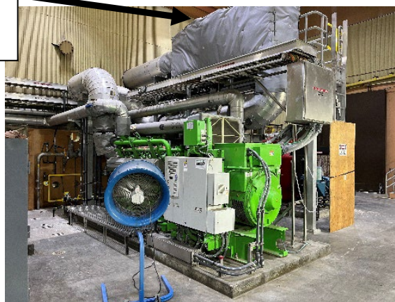
RTP Cogen SCR Ladder Out of Service Covered by Plywood
