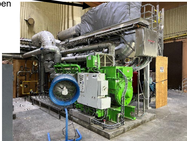
RTP Cogen SCR Ladder Out of Service Covered by Plywood
