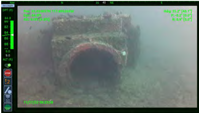
Entry 7 - Junction Box
