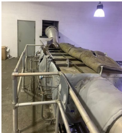
The JBL SCR has handrailing around the SCR to protect employees
