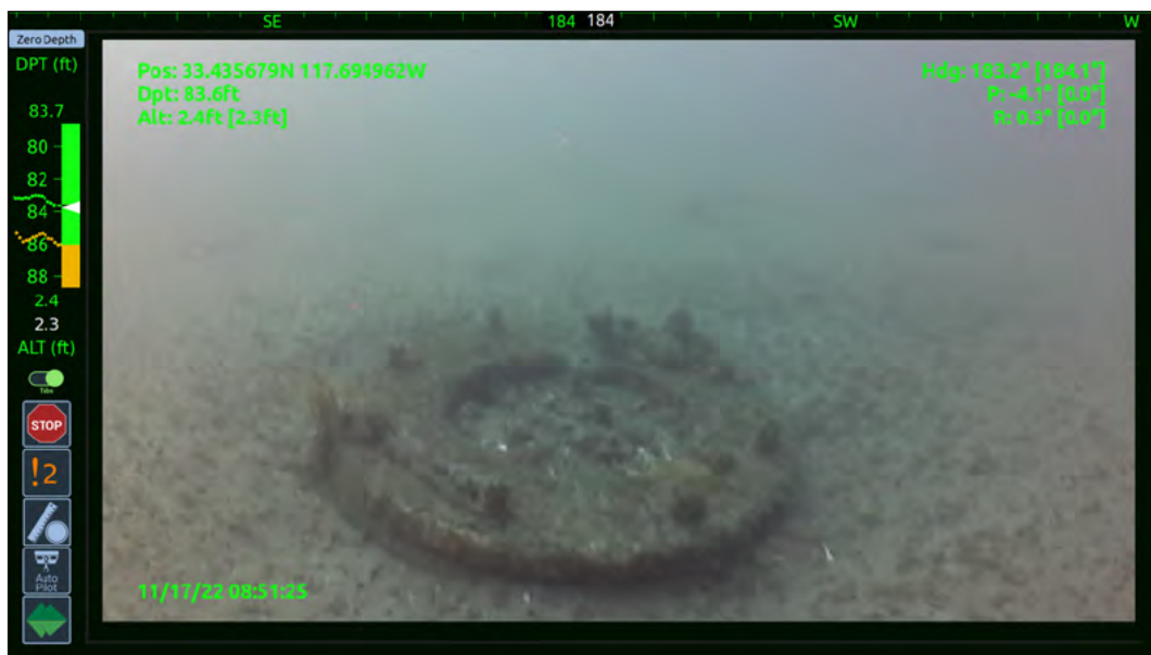
Photo 8 – View of an SJCOO outfall manhole, slightly protruding from beneath the sand
