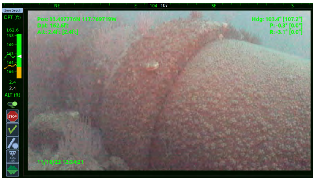
Photo 4 – View showing the typical condition of a bell joint at the ACOO
