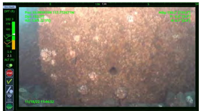
Entry 7 North diffuser not flowing
