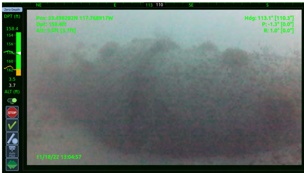
Photo 10 – View of an area along the ACOO that is missing ballast, well below the springline
