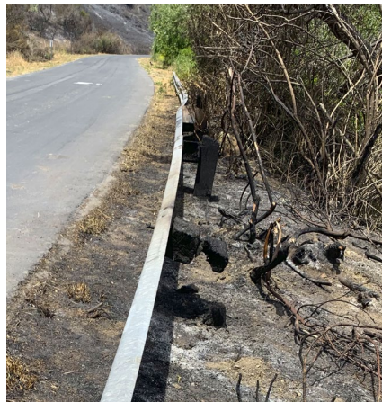
Figure 1: Fire Damaged Guardrail
