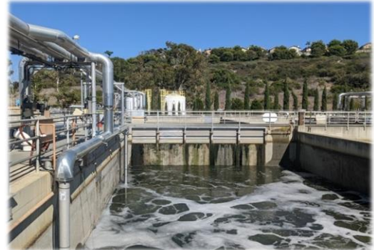
Regional Treatment Plant
