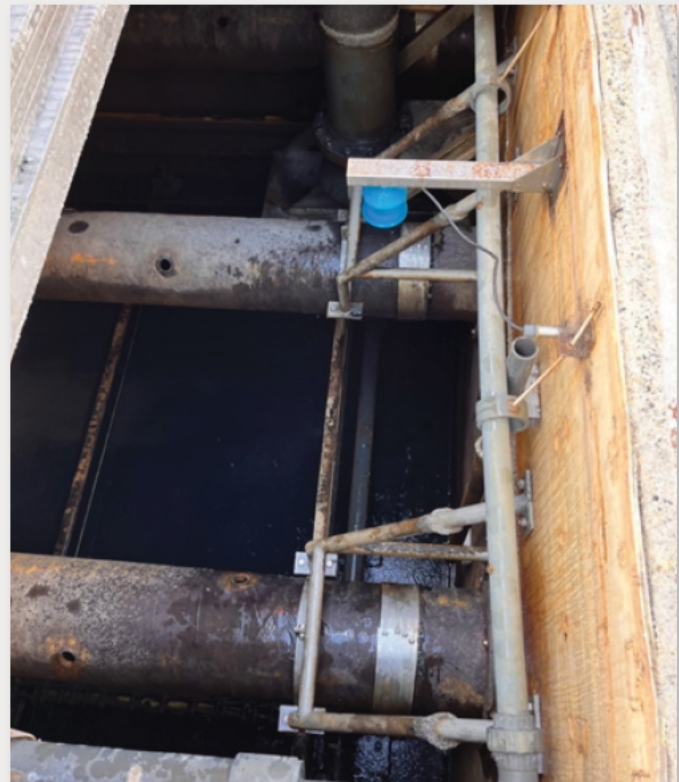
Figure 4. Primary Sedimentation Tank Effluent Pipes
