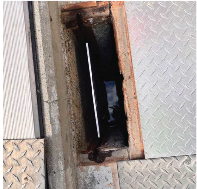
Figure 3. Slide plates are challenging to seat, especially in corroded slots. Replacing plates with manually operated slide gates eases operability of the system.
