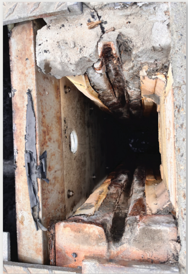
Figure 2. Primary Sedimentation Tank Slide Plate
