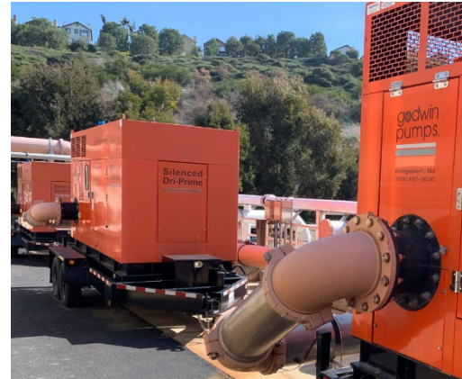
Temporary Bypass Pumps at SOCWA Regional Treatment Plant
