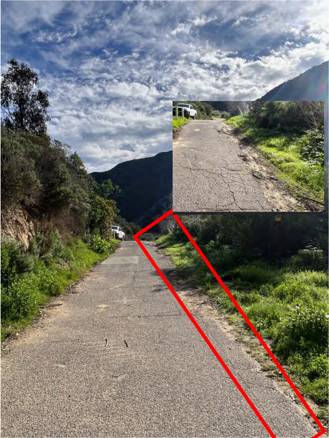
Sample area of continued road loss due to water erosion (in red square)
