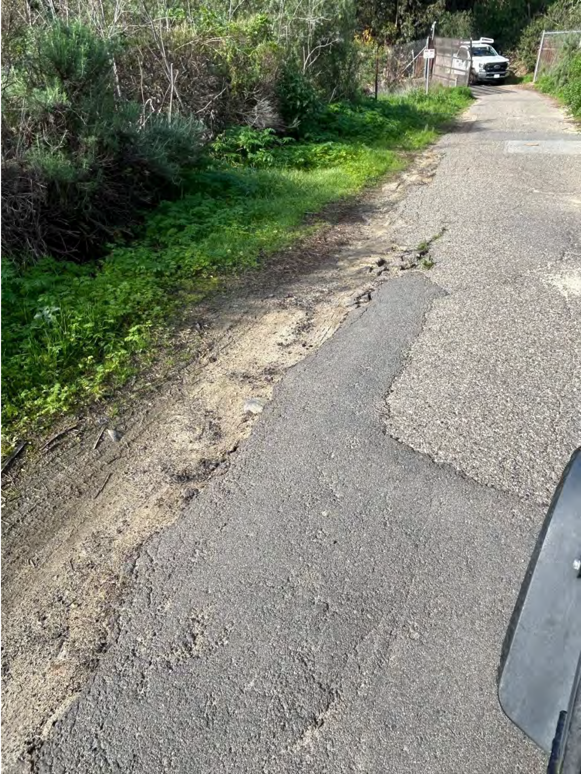
CTP Access Road Near Golf Course Entrance 1/2026 (sample area of repairs to up to 1/2 of the road was lost and repaired)
