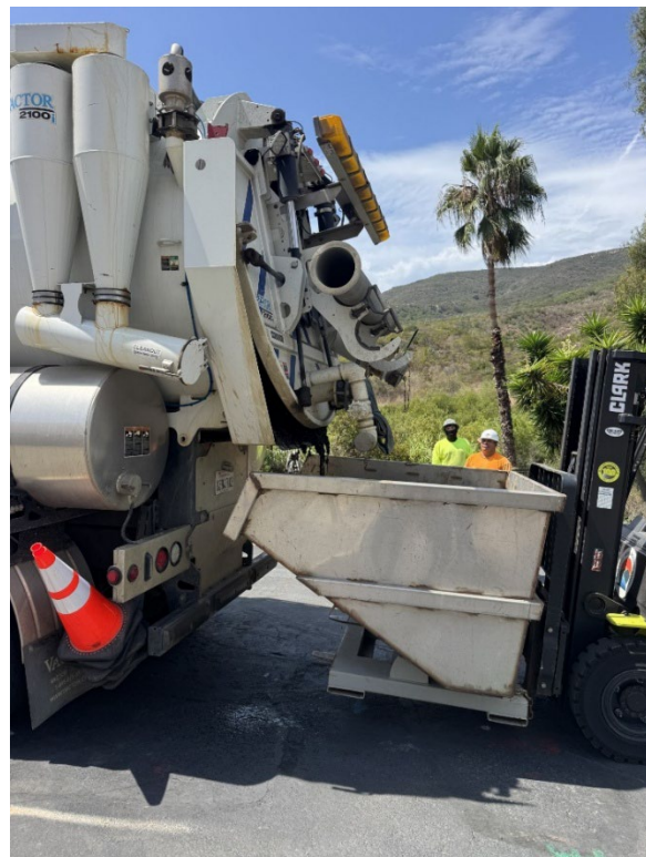
CTP Vactoring Primary Tank Hoppers
