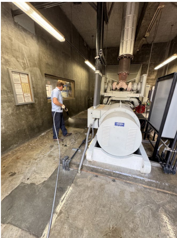
CTP Cleaning Engine Room
