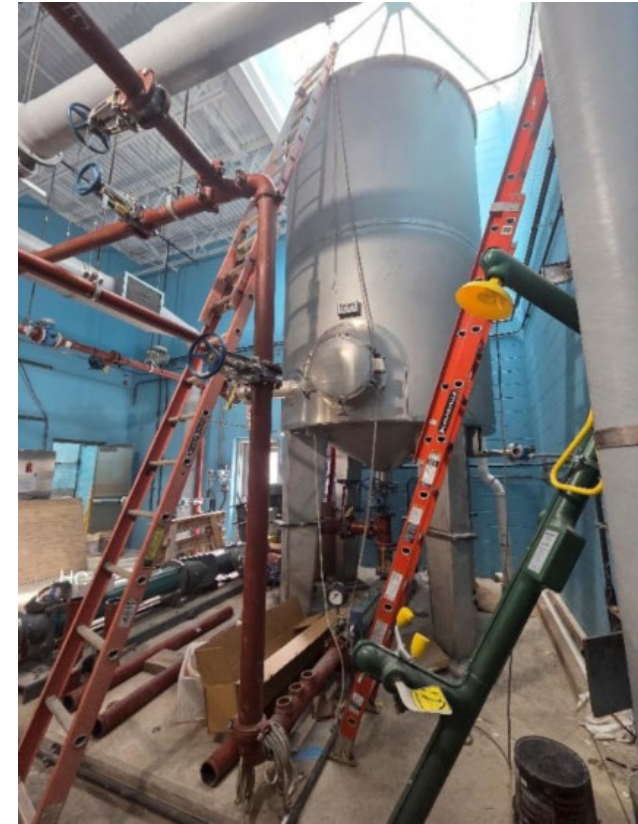
Thermal Chemical Hydrolysis Process (TCHP) Reactor
