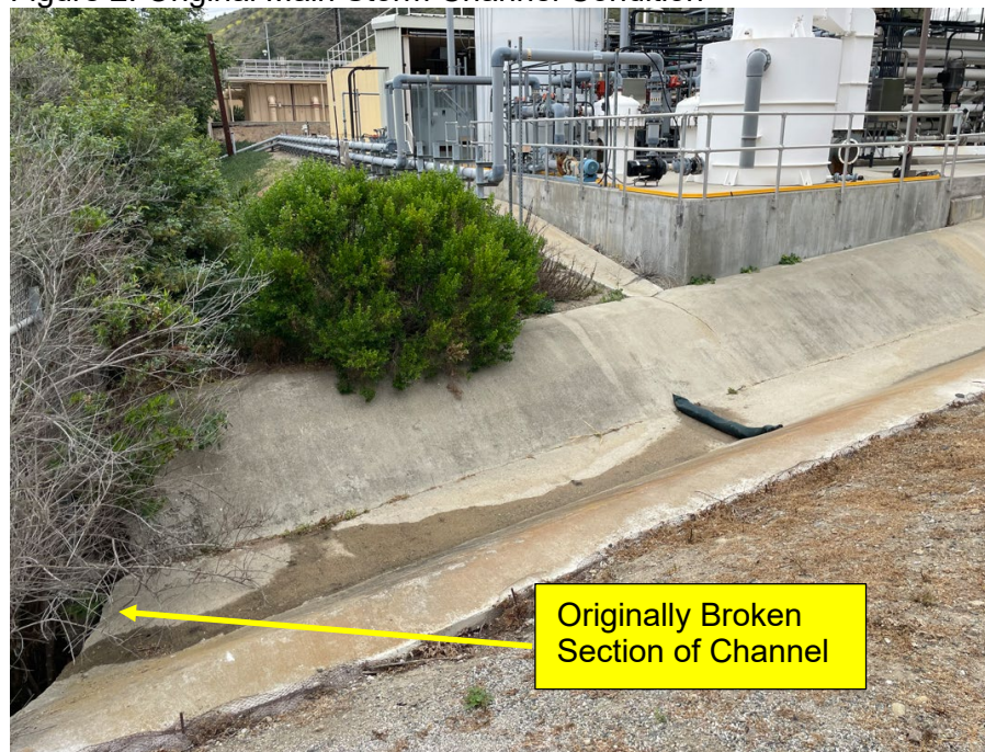
Figure 2: Original Main Storm Channel Condition
