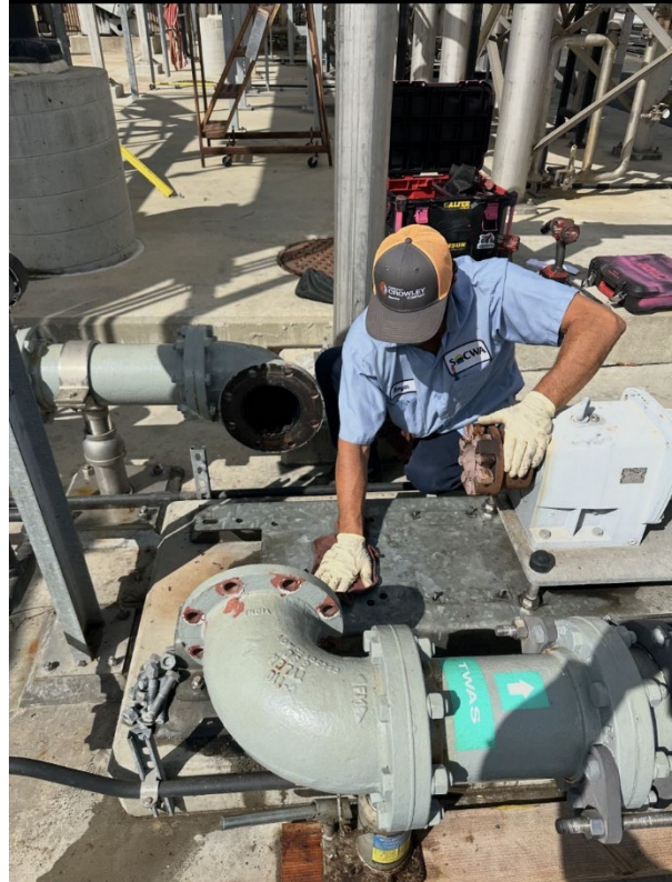
JBL TWAS PUMP REBUILD
