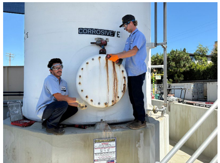
JBL RAS Bleach Tank Gasket Replacement
